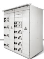
Low Voltage Switchgear & Motor Control Center
